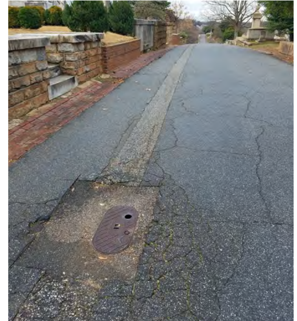
Watering system updates from 2000 with sinking asphalt patch.
