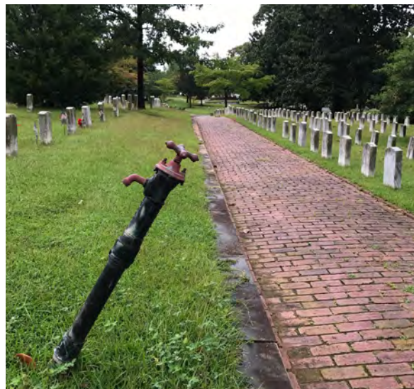
Old Murdock yard hydrants serviced most sections of the cemetery prior to new piping in the 1990s.
