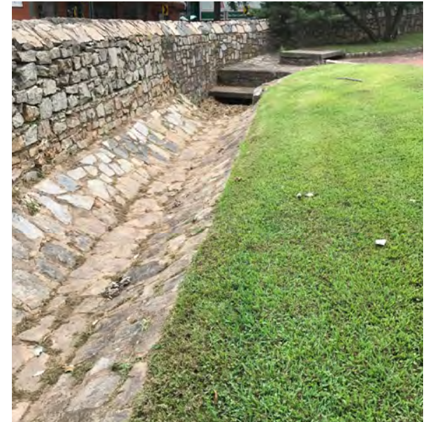
Shown as "LP-5" on the Stormwater map on page 109, this catchment structure was added in 2000 to reduce flooding in the southeastern edge of the Paupers Grounds. South of here is a proposed location for a cistern
