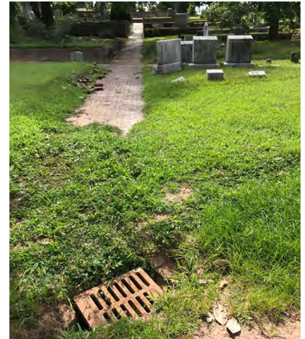
Standing water has allowed sediment to cover brick gutters, greatly reducing their functionality.
