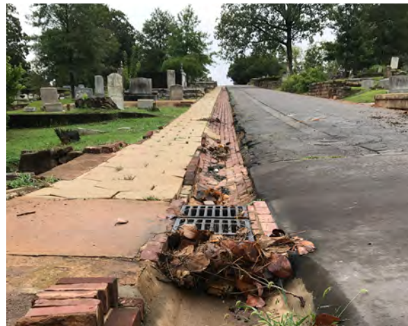
Debris blocks inlets in heavy precipitation events. Low points such as this provide green infrastructure opportunities.
